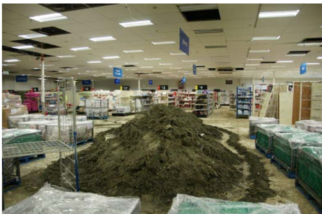
▼ Figures 8: Liquefaction silt at the Palms Shopping Mall
